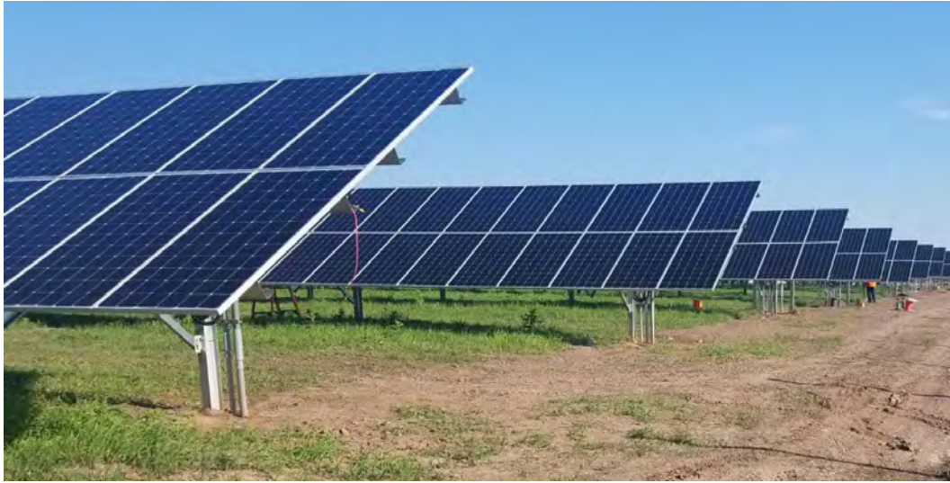
Fixed mount – (Alliant Energy, Fond du Lac, Wisconsin, USA)
