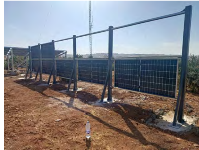
Vertical Panels – Under Construction at University of Jordan (Photo: Dr. Osama Ayadi, School of Engineering, University of Jordan)
